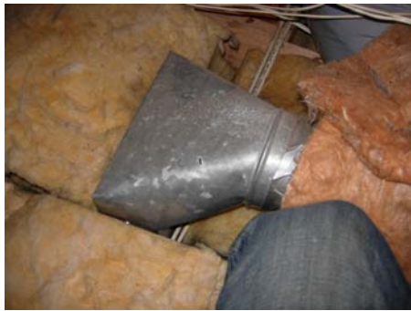
5. Leaky boots (using duct tape)
