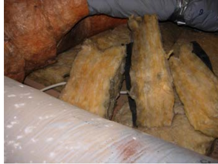
2. Poorly installed insulation on attic floor
