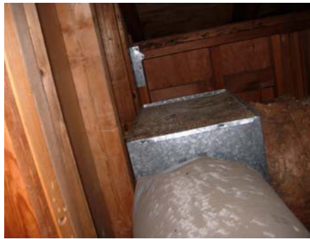
6. Uninsulated a leaky return plenum
