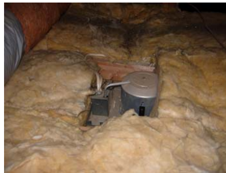
4. Fiberglass touching recessed light
