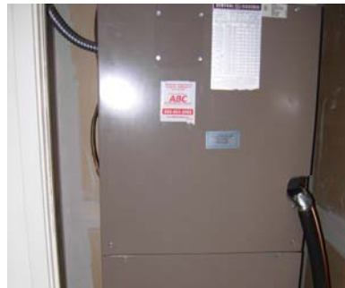
8. Electric furnace for primary heating
