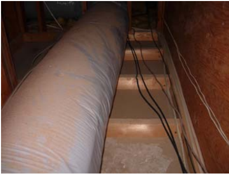
1. Missing Insulation on attic floor
