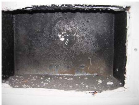
7. Looking inside very dirty duct register
